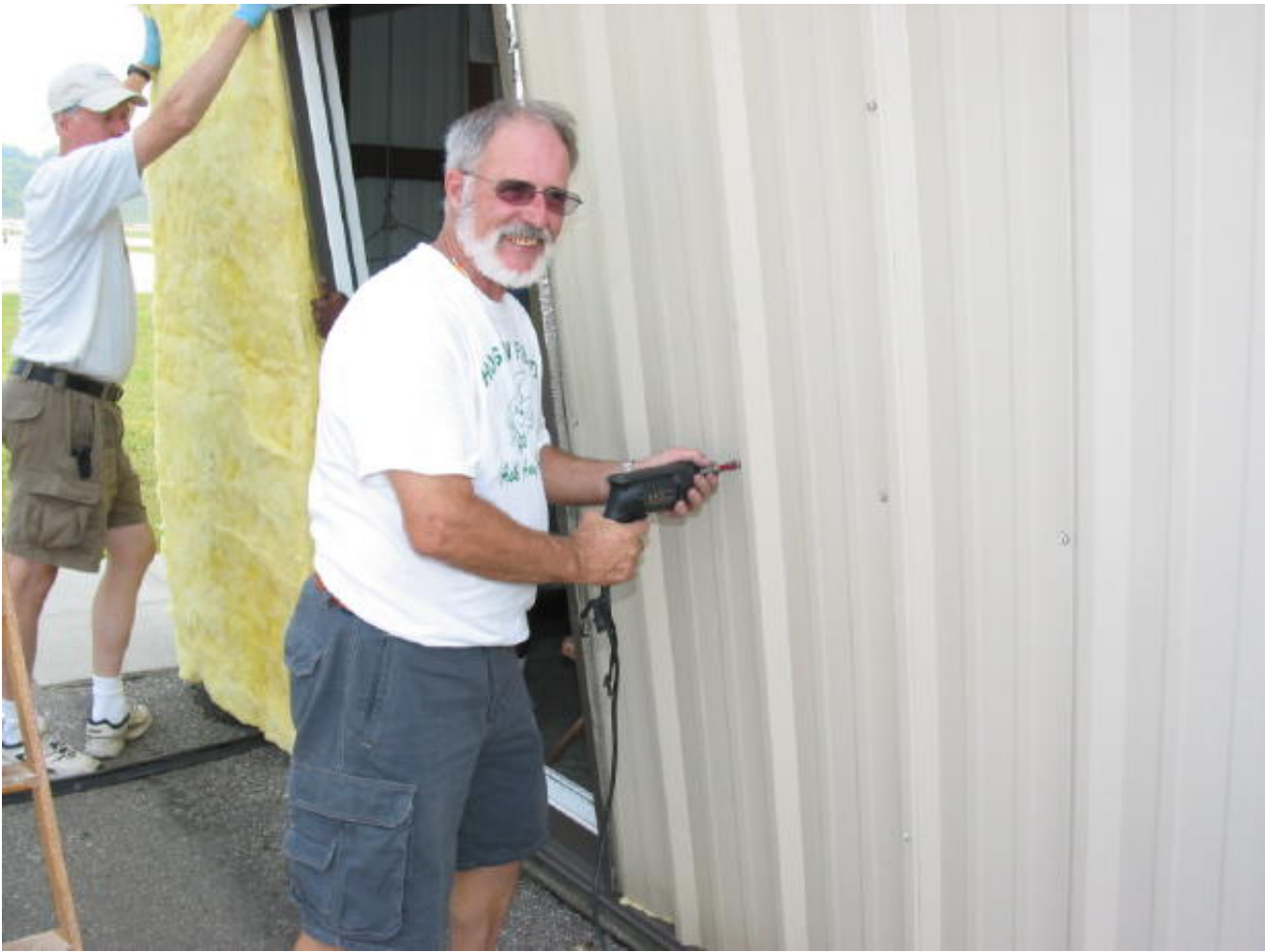
Is that a drill? Look where you're drilling people!
